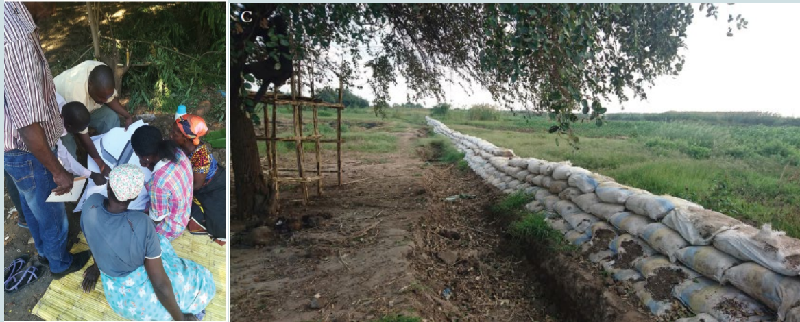
Figure 15: Villagers discussing dyke design with consultants in GVH Nafafa in Malawi and dike construction (Van Den Homberg and Sadik Trogrlic, Robert, 2023)
